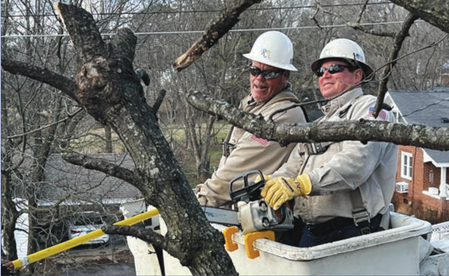
David Deloach, left, and Bill Newman work together to trim back trees and other vegetation away from power lines.
