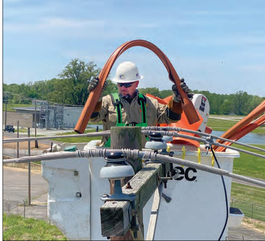
Always working with safety in mind, Lineworker Chris Sanders puts insulated tubing on a power line before starting work.
